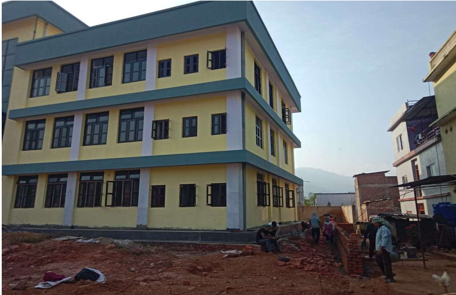
Divyajyoti Secondary School, Mathgadhi-03, Palpa
